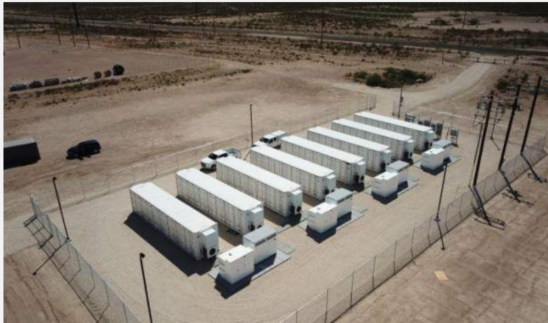
Photo 2: Aerial view of a typical BESS Project site.
